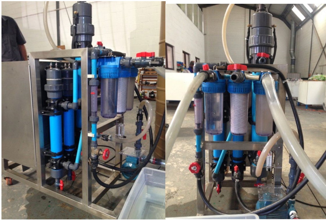
Photograph 3 & 4: Shows the EMAWS Water Treatment System with the larger Electro-Coagulation Reaction Cell on the right, and the two smaller Electro-Oxidation Cells on the left. In front of the Reactions Cells are the sight-glasses for each step, with the 50 Micron Polishing Filter installed between the two sight-glasses.
