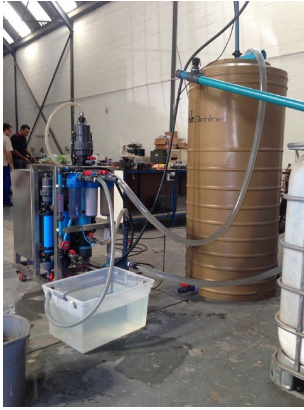
Photograph 1: Shows the EMAWS System with the Treated Electro-Oxidized Water Collection Tank in the foreground and the 0.75m 3 Electro-Coagulation Clarifying Tank on the right. The Electro-Coagulated Sludge discharge line can also be seen discharging into the Sludge Collection vessel (partial view in right foreground).
